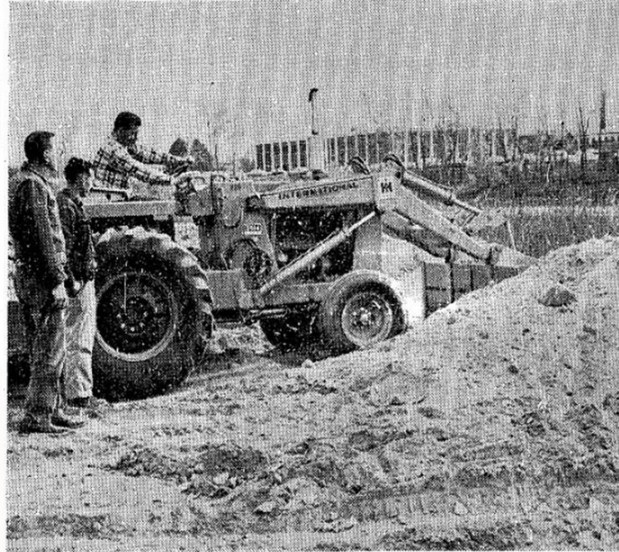
BROWN DIRT that will serve next spring as the foundation for Boise's first section of the Green Belt is leveled under the supervision of Boise City park men. Clay Wilson, crew foreman, operates the tractor. Looking on are Park Supervisor Gordon Bowen, left, and Skip Gates, the Julia Davis foreman. The work on this section of the Green Belt extends about a quarter-mile east of the Capitol Boulevard Bridge.
